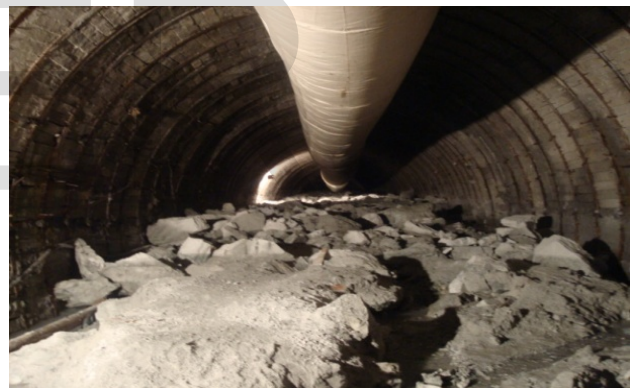
Photo:6: Cavity /blowout ch: 616.68m in HRT Face-II
