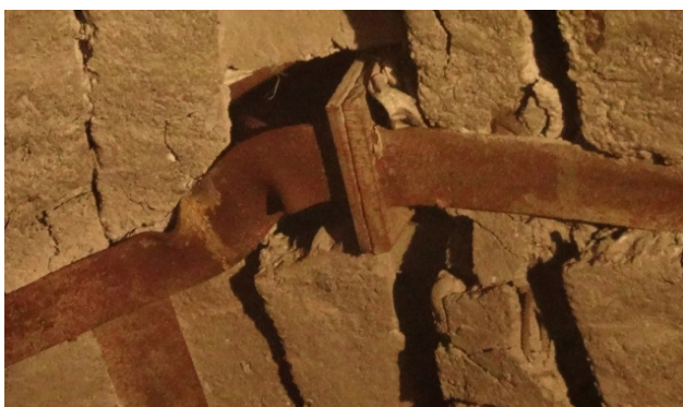
Photo: 8 Squeezing Rock strata in HRT Face-III
