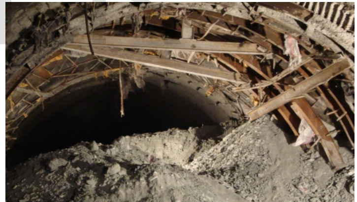
Photo:10 The face condition where the dry crushed sheared material suddenly comes out exerting high pressure in rib support. Ch: 1385.0m, HRT Face-III.
