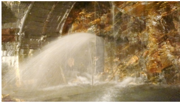
Photo: 11: The seepage water comes out at high pressure.
