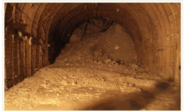
Photo: 5: Cavity /blowout ch: 422.6m in HRT Face-II
