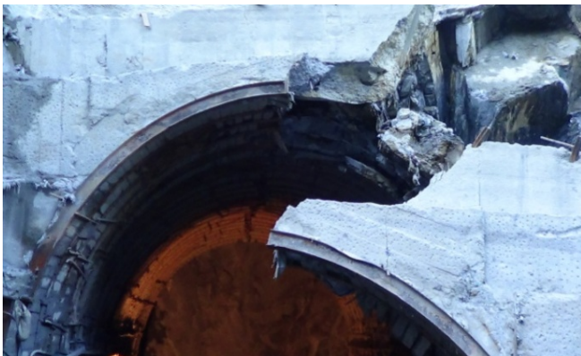
Photos: 4: Shear failure of steel rib due to developed stresses in cut and cover portion above the flash portal & cavity formation.
